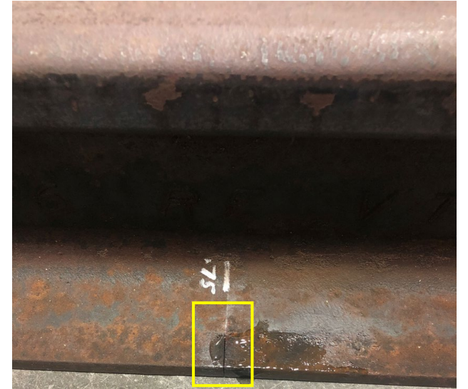
Rail showing notch in the base
