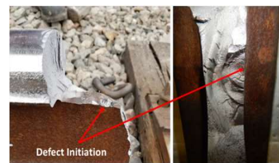
EFB weld failure at 210 MGT
