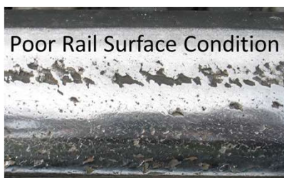
Rolling contact fatigue (RCF) damage
