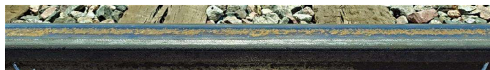
Severe RCF with spalls at end of test (654 MGT) on top of rail surface in type A low rail
