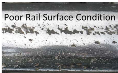
Rolling contact fatigue (RCF) damage
