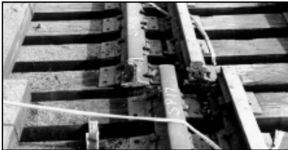
Exhibit 2. Lateral Displacement with Rails Cut
