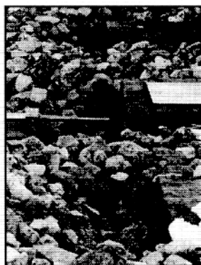
Closeup view of tie end showing shift of several inches.
