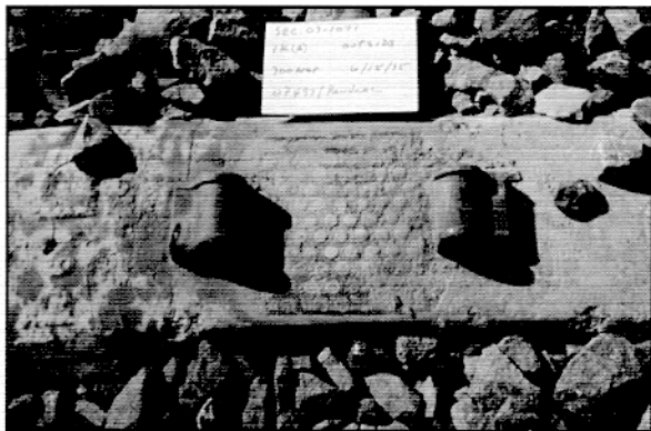
Exhibit 1. Appearance of Rail Seat Abrasion in the Field
