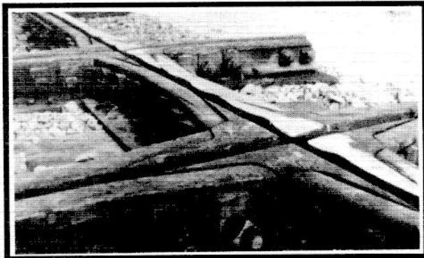
Exhibit 1. 89-Degree Crossing after 1.9 MGT of HAL Traffic
