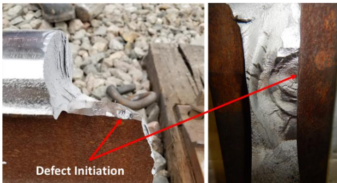
Figure 5. EFB weld failure between test rails
