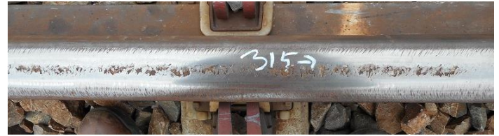
Figure 4. RCF on HS low rail in western revenue service site
