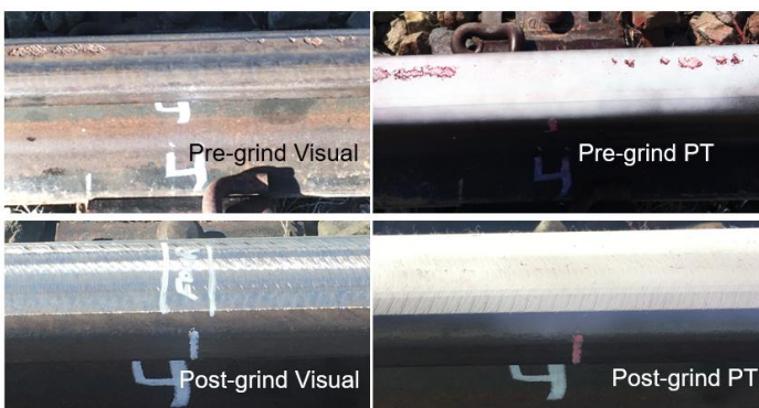
Figure 6. Pre- and post-grind visual and PT measurement for Location 4
