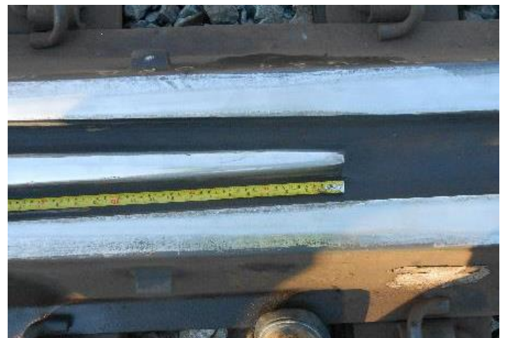
Figure 4. Running surface condition of weld repaired frog near 5/8-inch point
