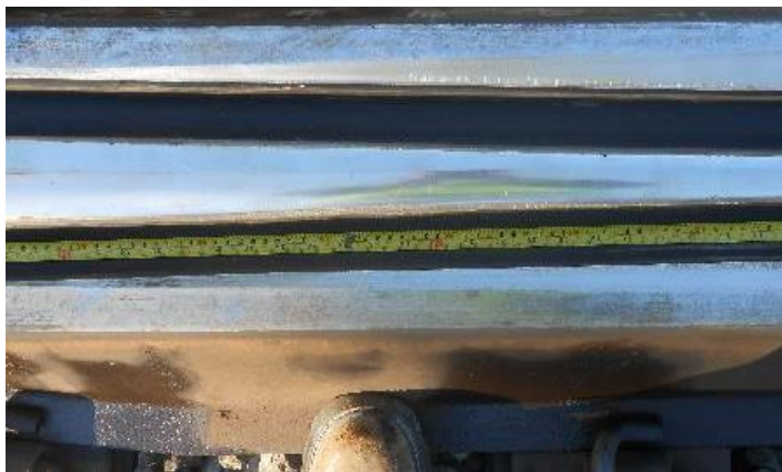
Figure 5. Running surface condition of weld repaired frog towards heel end of wheel transition zone
