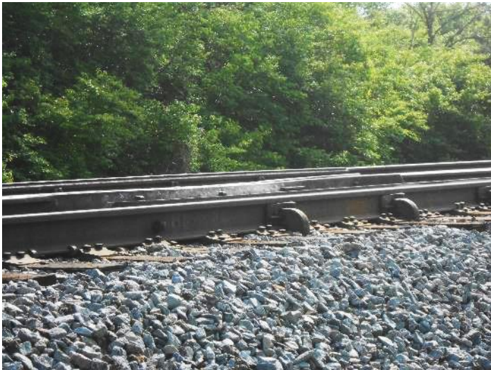
Figure 9. Repaired frog in-track showing bowed shape
