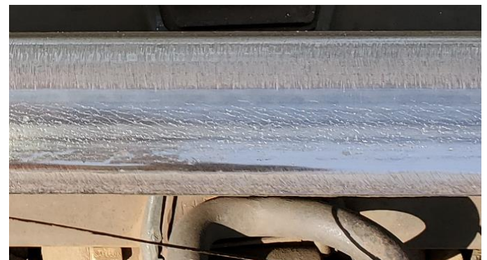
Figure 5. Location No. 28 on low rail during May 2019 inspection
