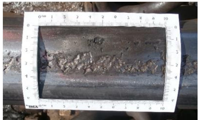
Figure 4. RCF, location No. 28 on low rail during April 2016 inspection
