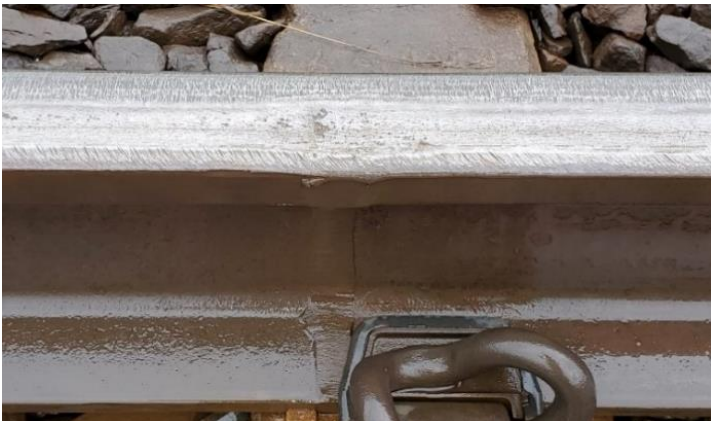
Figure 9. Rail batter development on electric flash butt weld
