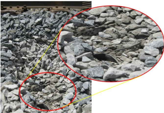
Figure 6: Geocell exposure showing fines infiltration
