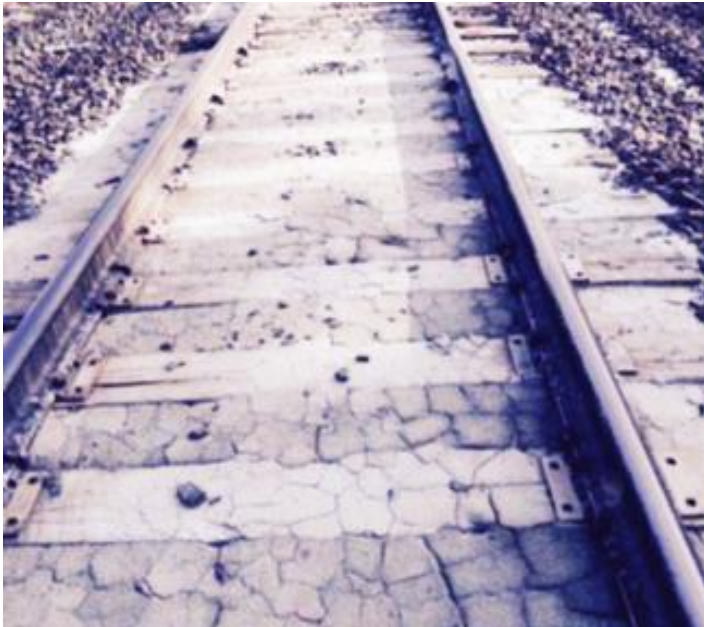
Figure 1. Fine-filled ballast from mud pumping
