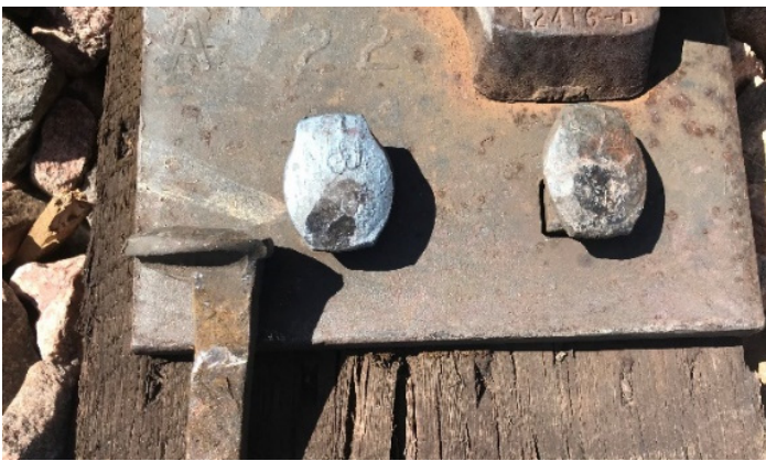
Figure 2. Broken spikes on 18-inch elastic fastener plates (Zone 5)
