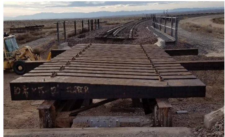
Figure 3. Superelevated glulam ties installed on a 30-foot DPG span in the State of the Art (SOA) Bridge at FAST
