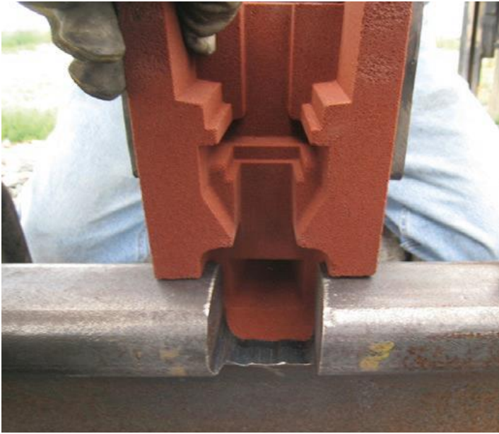
Figure 1. Typical cut of the rail head during the rail head repair welding process
