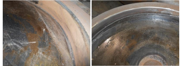
Figure 5. Horizontal wear liner condition with original lever plate (l) and modified center plate (r)
