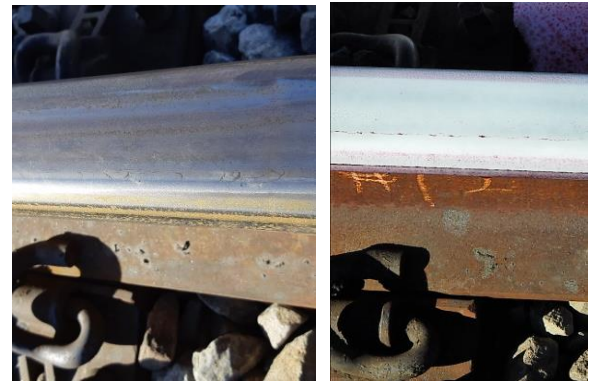
Figure 9. Visual and PT result for the high rail in HTL Section 7, 38 feet
