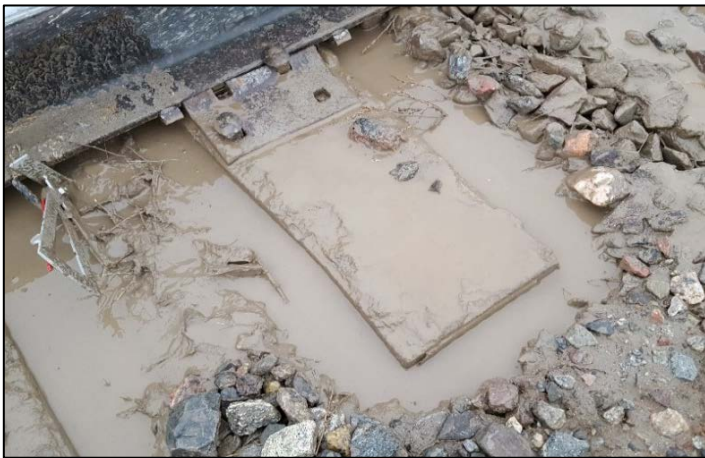
Figure 2. Photograph of mud pumping with standing water
