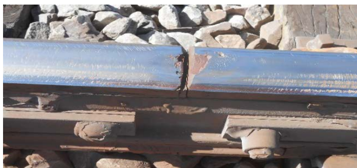
Figure 2. Rail end chipping on a butt jointed IJ
