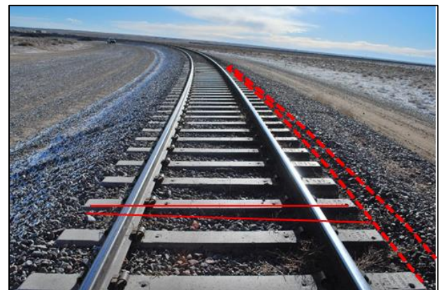
Figure 3. Typical ballast migration observed in Zone 2 (UTP 1)
