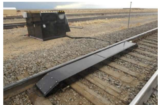
Figure 2. Complete assembly of RLL installed at FAST
