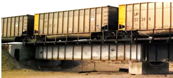
Figure 1. A 65-foot riveted deck plate girder span in the East Steel Bridge at FAST
