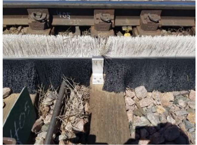
Figure 1. Brush System Installed with Holding Bracket
