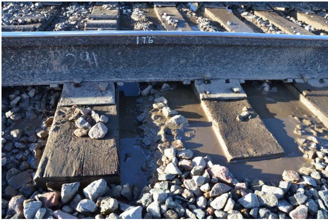
Figure 3. Mud Pumping after 4th night (10/11/2017)
