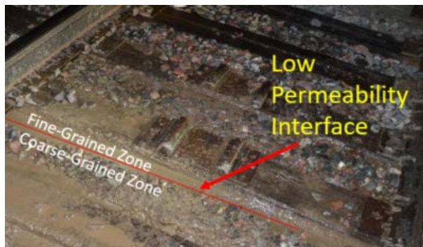
Figure 5. Photograph of Mud Pumping in the Rainy Section
