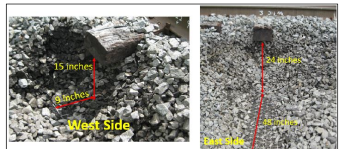
Figure 9: Exposed geogrid measurements showed migration downward and to the east
