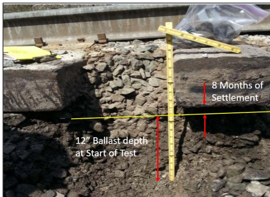
Figure 6: In early 2013, 0.10-foot of ballast settlement was already evident
