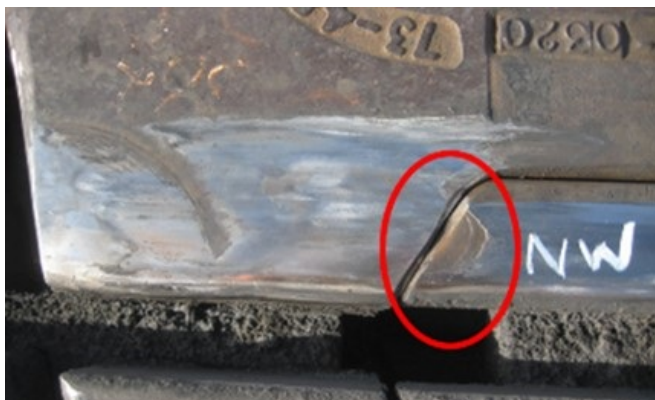
Figure 4. Rail chip at the NW corner developed during the 38 MGT bolt test
