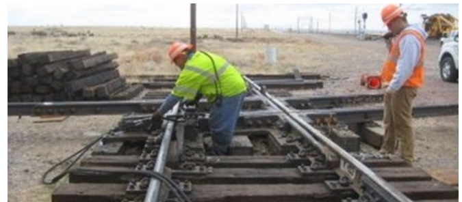
Figure 2. Crossing diamond being disassembled out of track for detailed inspection of components
