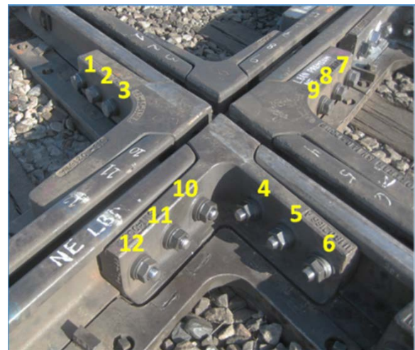
Figure 2. Typical 12-bolt configuration at each corner of the crossing diamond, NE corner shown. Traffic ran in both directions along the 1 through 6 bolt line.
