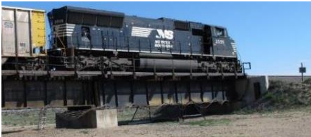
Figure 1. 55.5-foot Riveted Deck Plate Girder Span in the East Steel Bridge at FAST
