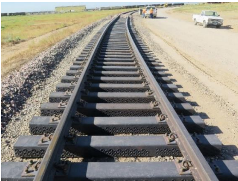
Figure 1. Skeletonized EPC Tie Zone during Installation before Ballast Dumping. Note Texturing on Sides of Ties
