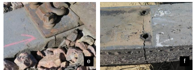
(e) and (f) Spike hole cracks in drive spike holes
