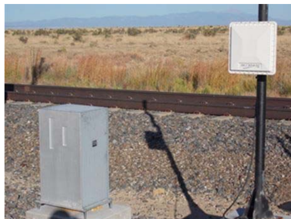
Figure 2. TFDS rail side camera box and AEI reader
