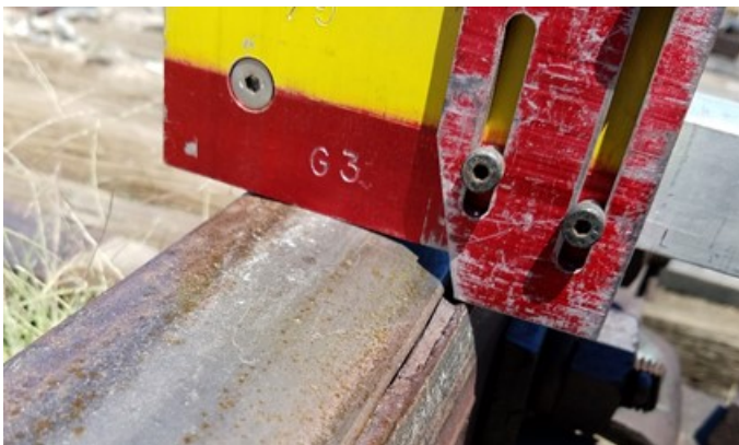
Figure 3. Gauge Caught on Condemnable Worn Switchpoint
