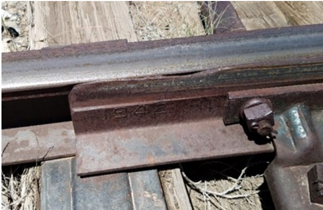
Figure 2. Worn Switch Point Inspected Using NS Gauges
