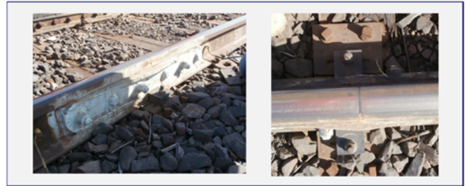
Figure 9. L. B. Foster Endura-Joint at 75 MGT
