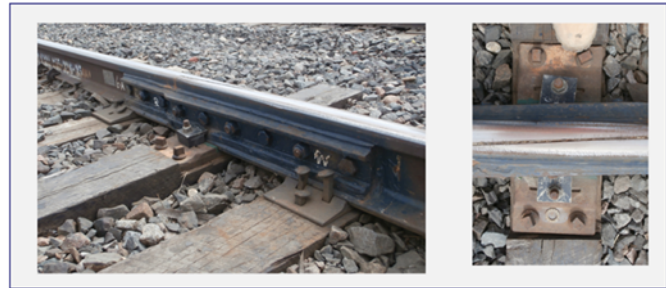
Figure 10. Koppers Short Angle Projection Joint at 65 MGT
