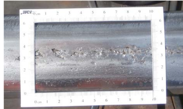
Figure 6. Example of Low Rail Surface Condition ~30 MGT since Grinding
