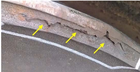
a. Shattered Rim Crack
