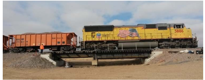
Figure 1. 24-foot and 32-foot Riveted DPG Spans in the West Steel Bridge at FAST
