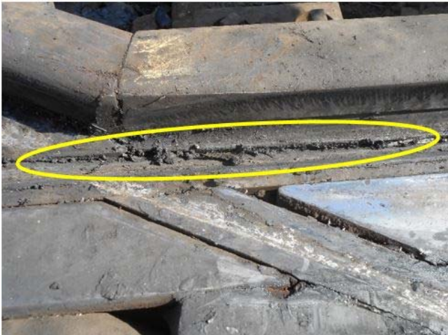
Figure 2. Cracked Flange Bearing Bar Associated with Non-centered Running
