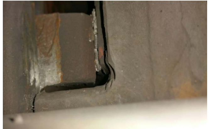
Figure 7. Magnets on the Other Side Fractured
