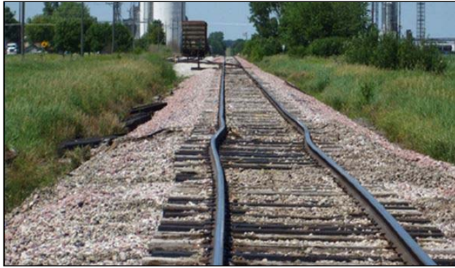
Figure 1. Photograph Showing Thermally Induced Buckling of a Rail Structure
