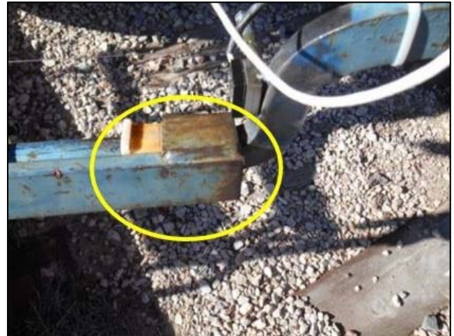
Figure 5. Insert Slipping from Designed Position
