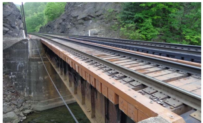
Figure 5. Bridge Tie Test on 67-foot Girder Span at the Eastern Mega Site
