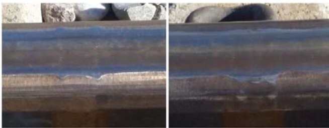
Figure 9. (Left) Surface photo of an untreated test weld (Right) Surface photo of a HAZ treated test weld
