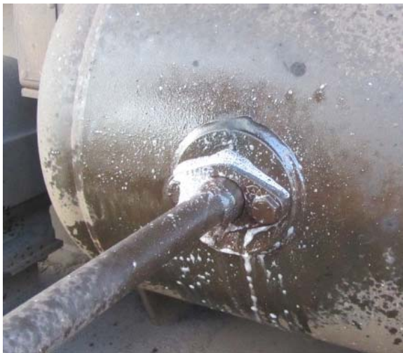
Figure 2. Auxiliary Flange Leak Indicated by Leak Detection Fluid
