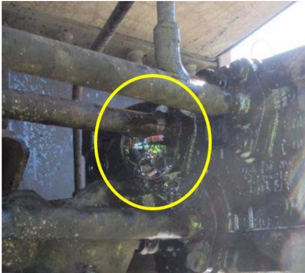
Figure 3. Larger Leak between Flange and Pipe Bracket Highlighted by a Yellow Circle
