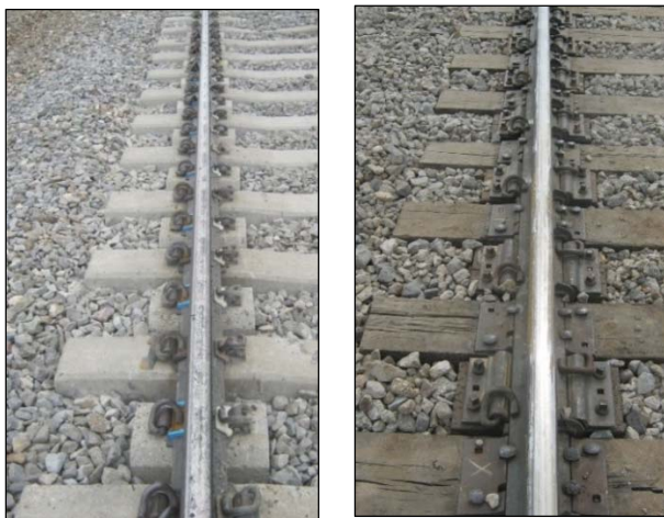
Figure 4. (left) Concrete Crib Ties and (right) Wood Crib Ties at FAST
