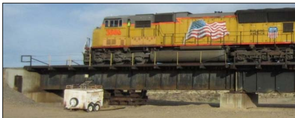
Figure 3: Full-time SHM system installed on steel girder span
