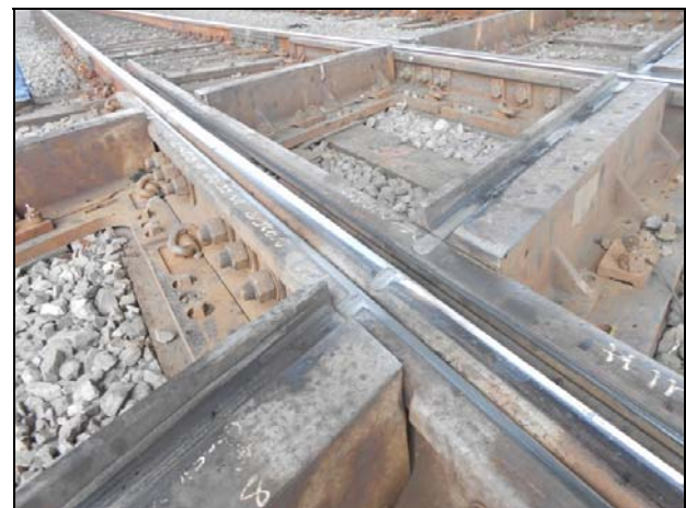
Figure 2. OWLS FBF Diamond at DT Junction, CA The flanges of crossing traffic run on the top of the mainline rails.
