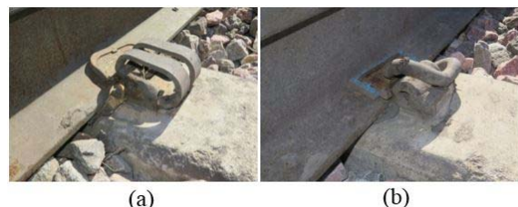
Figure 5. (a) A Common Insulator Failure on a McKay type fastener in Zone 5 and (b) A Common Insulator Failure on an e-clip type fastener in Zone 2.
