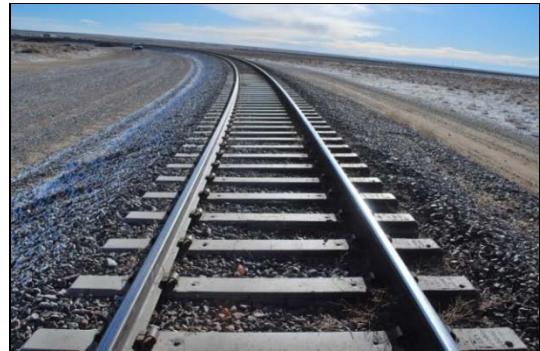
Figure 4. Typical ballast migration observed in Zone 3, reducing the lateral restraint provided by the high rail shoulder
