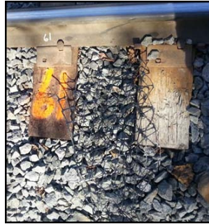
Figure 7b. Geogrid may be damaged during shoulder cleaning
