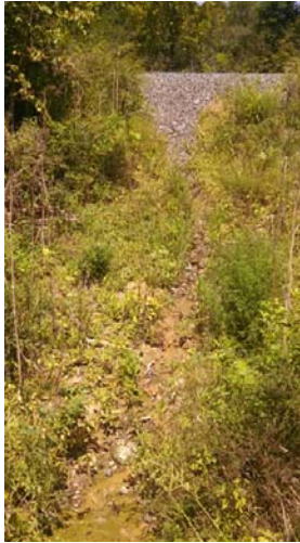
Figure 7a. Ballast drains still functioning in 2014, but appear to be slowing down
