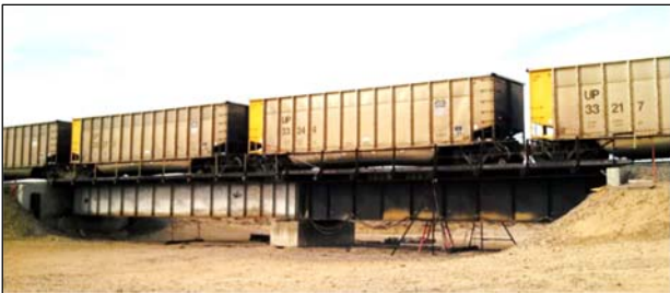
Figure 1. FAST Steel Bridge with 65-foot and 55.5-foot Riveted Deck Plate Girder Spans
