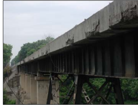
Figure 2. 55.5-foot Riveted Span (second span from camera) in Prior Service with Concrete Floor and Ballast Deck
